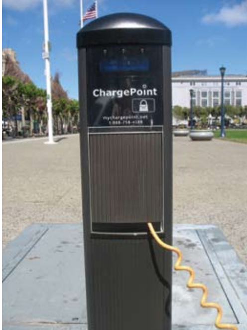
On-street car chargers, like this one in San Francisco, will make it easier for people who don't have off-street parking to own plug-in cars. Photo credit: Siena Kaplan.
