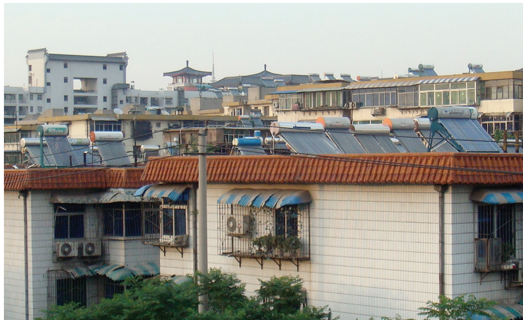
Rooftop solar collectors supply hot water to tens of millions of households in China. Here, solar collectors line rooftops in the city of Xi'an. Photo Credit: Kerry Snyder
