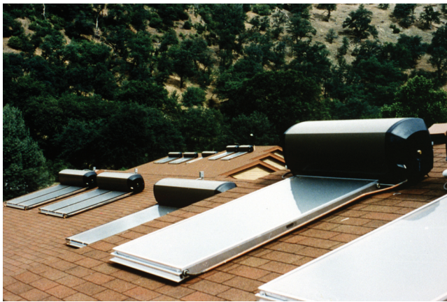
Solar water heaters on employee housing in Yosemite national park Courtesy of DOE/NREL, Credit: Jim Schwerm
