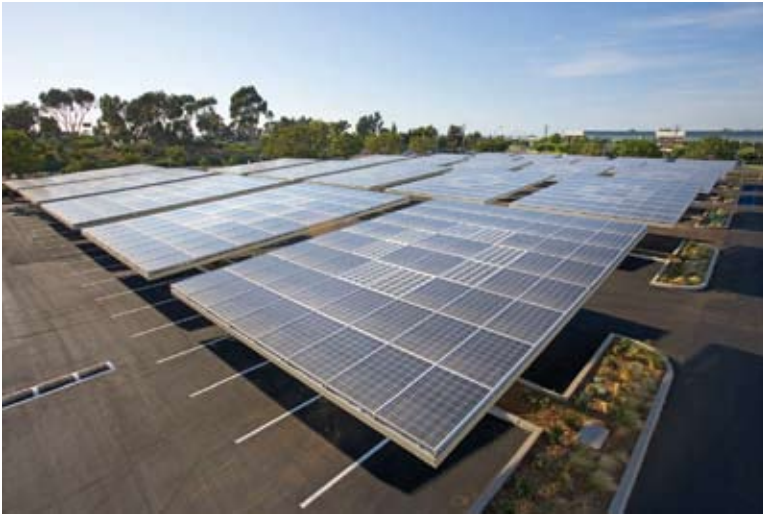
With “vehicle to home” technology, plug-in car owners could charge their cars during the day at solar parking lots—such as this one at Kyocera’s employee parking lot in San Diego, California—then use remaining battery power after they drive home to help power their houses in the evening. Photo credit: Envision Solar.
