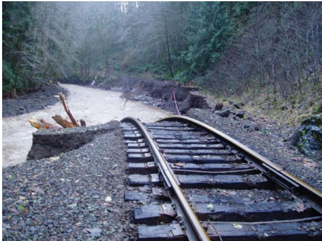
Floodwaters washed out a rail line in the Pacific Northwest during the destructive December 1-3, 2007 winter storms that pounded the Pacific Coast. Credit: National Weather Service
