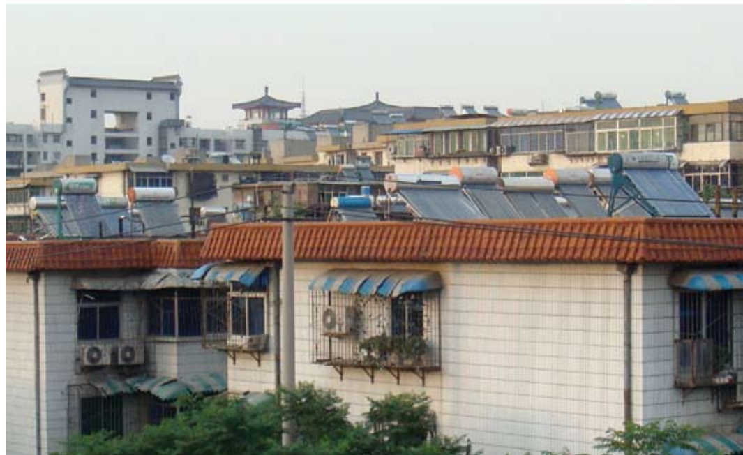
Rooftop solar collectors supply hot water to tens of millions of households in China. Here, solar collectors line rooftops in the city of Xi'an. Photo Credit: Kerry Snyder
