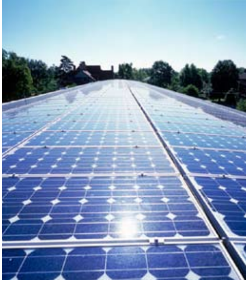
Solar photovoltaic (PV) panels transform sunlight into electricity.
