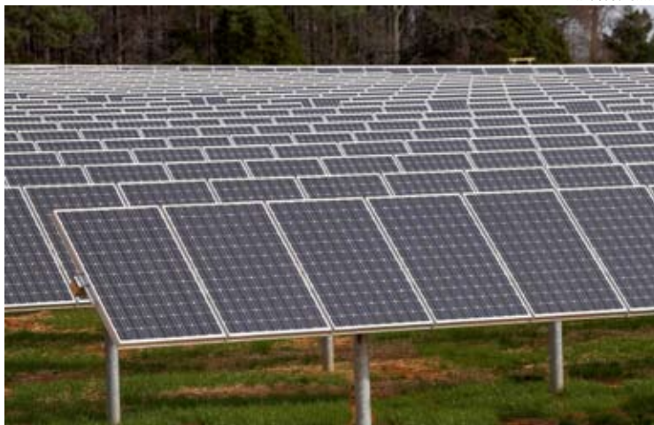
SAS installed a 1-megawatt solar farm on the campus of its world headquarters in Cary in 2008. SunPower designed the facility and Southern Energy Management installed it.
