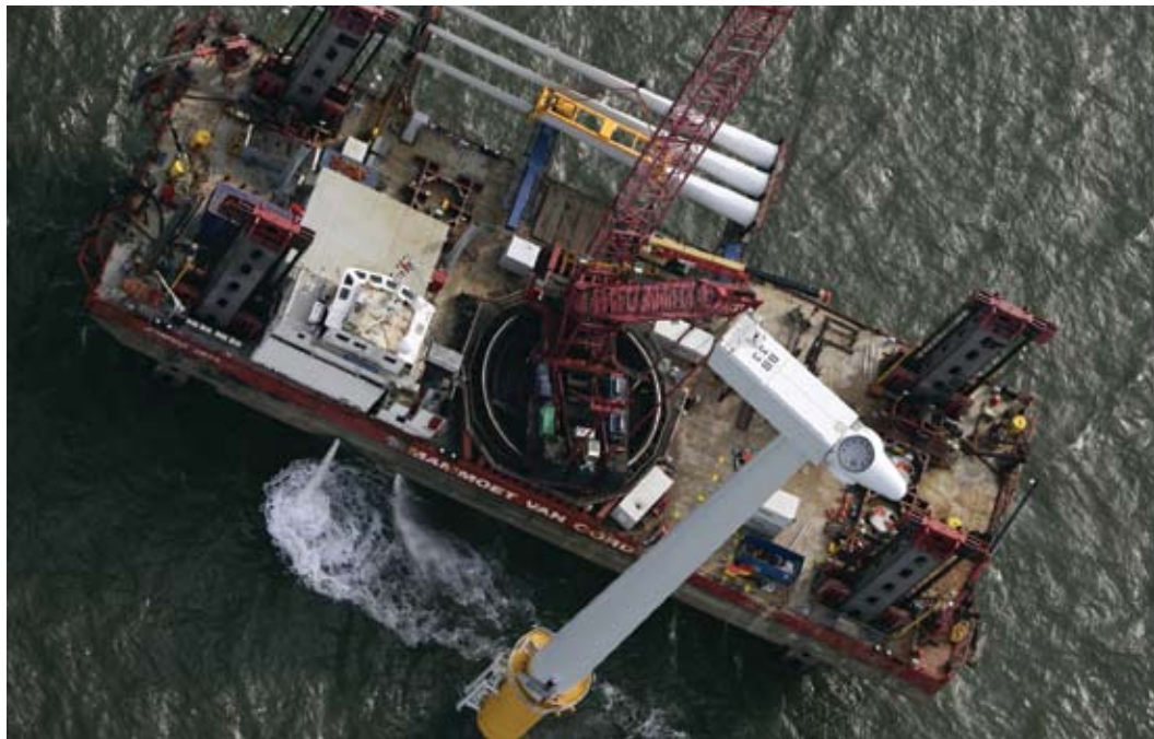
Installation of offshore wind turbines requires the use of specialized ships—such as the jack-up barge pictured above—equipped with massive cranes. The three rotors of the wind turbine under construction above can be seen on the far side of the jack-up ship. Credit: Siemens.
