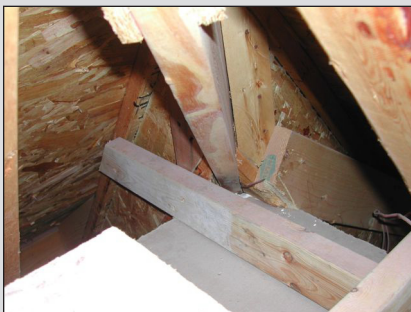
Improper Roof Construction: Two inspection firms, including one that produces the products used in the Gilbert's roof, concluded that the roof is so poorly attached to the rest of the house that it is unsafe to live in.
