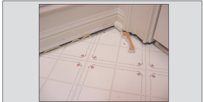
The Richardsons discovered that their foundation was sinking when the floors began to separate from the walls. The small piece of wood in the photo was inserted by the builder, Marbet Homes, during construction, suggesting that they attempted to use band-aid fixes to mask the larger problem.
