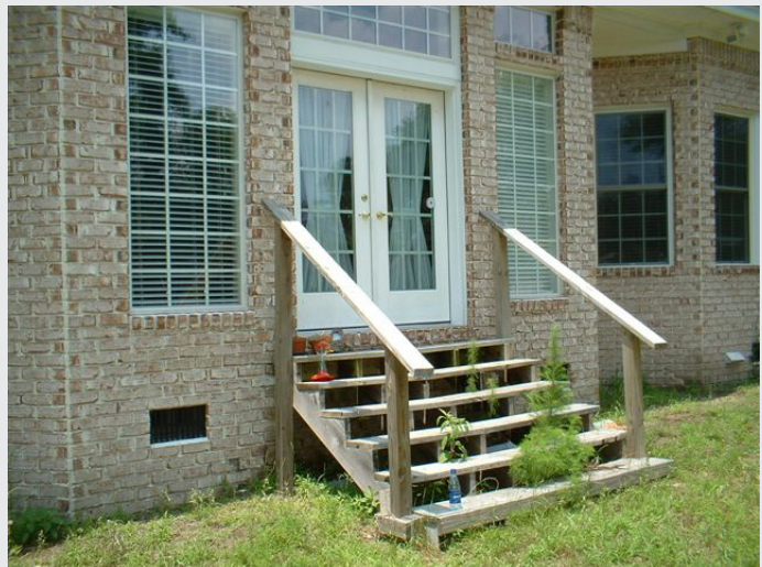
Careless Construction: These construction stairs were left on the back of the Gilbert’s house after the home was completed. These stairs are one of 31 code violations missed by the county inspector.
