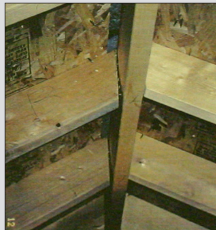
Roof rafters improperly cut to allow full bearing
