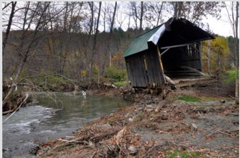
Flooding rains from Hurricane Irene destroyed roads and bridges throughout Vermont. The historic Bowers covered bridge (above), built in 1919, was lifted off its abutments and carried 200 feet downstream.
