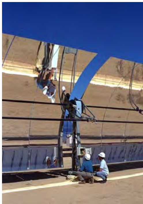
Technicians inspect the local controller on a parabolic trough array at Kramer Junction, California. (Credit: Gregory Kolb, Sandia National Laboratories)
