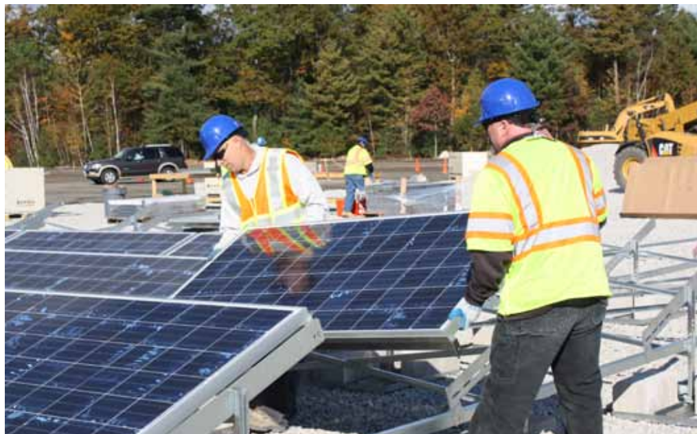
Workers install solar panels at a solar energy park in Westford – one of many new solar energy projects installed across Massachusetts in recent years.
