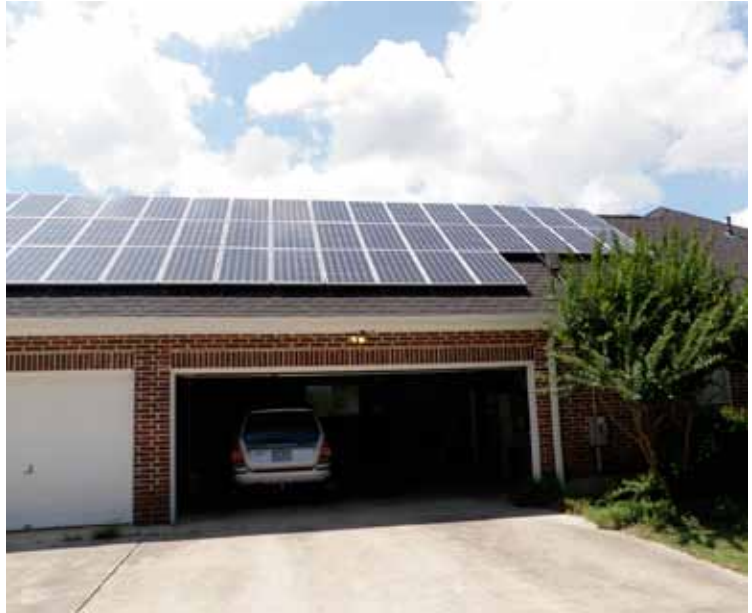
A solar energy system installed on the roof of a house in San Antonio with the help of CPS Energy.
