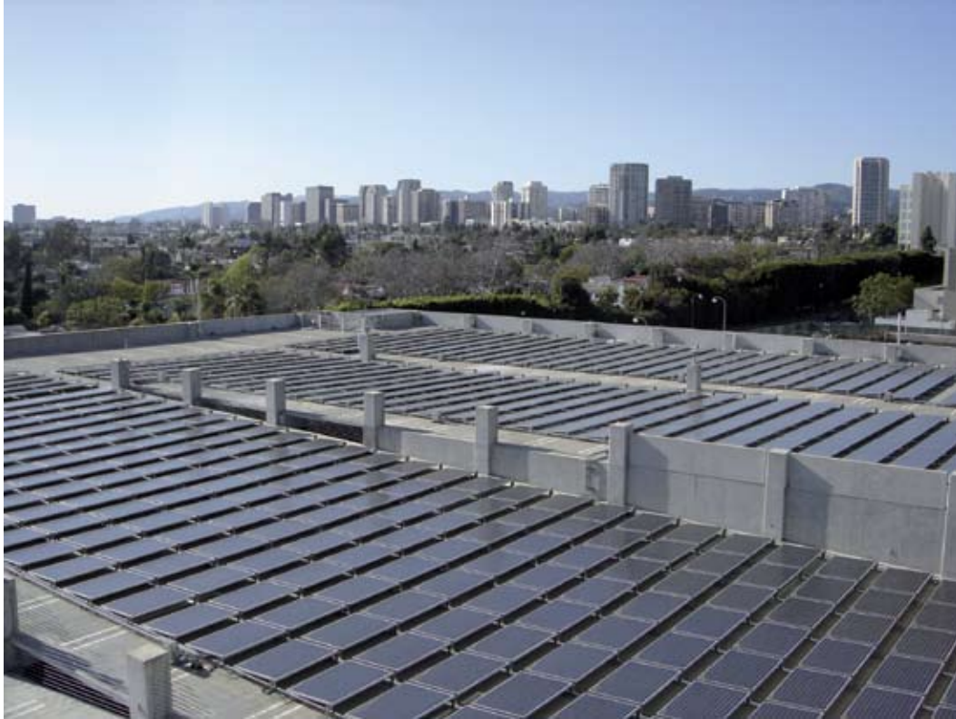
Constellation Place, a high-rise building in Century City, hosts a 1 MW solar array, saving approximately 100,000 per year. Credit: Environment California Research & Policy Center
