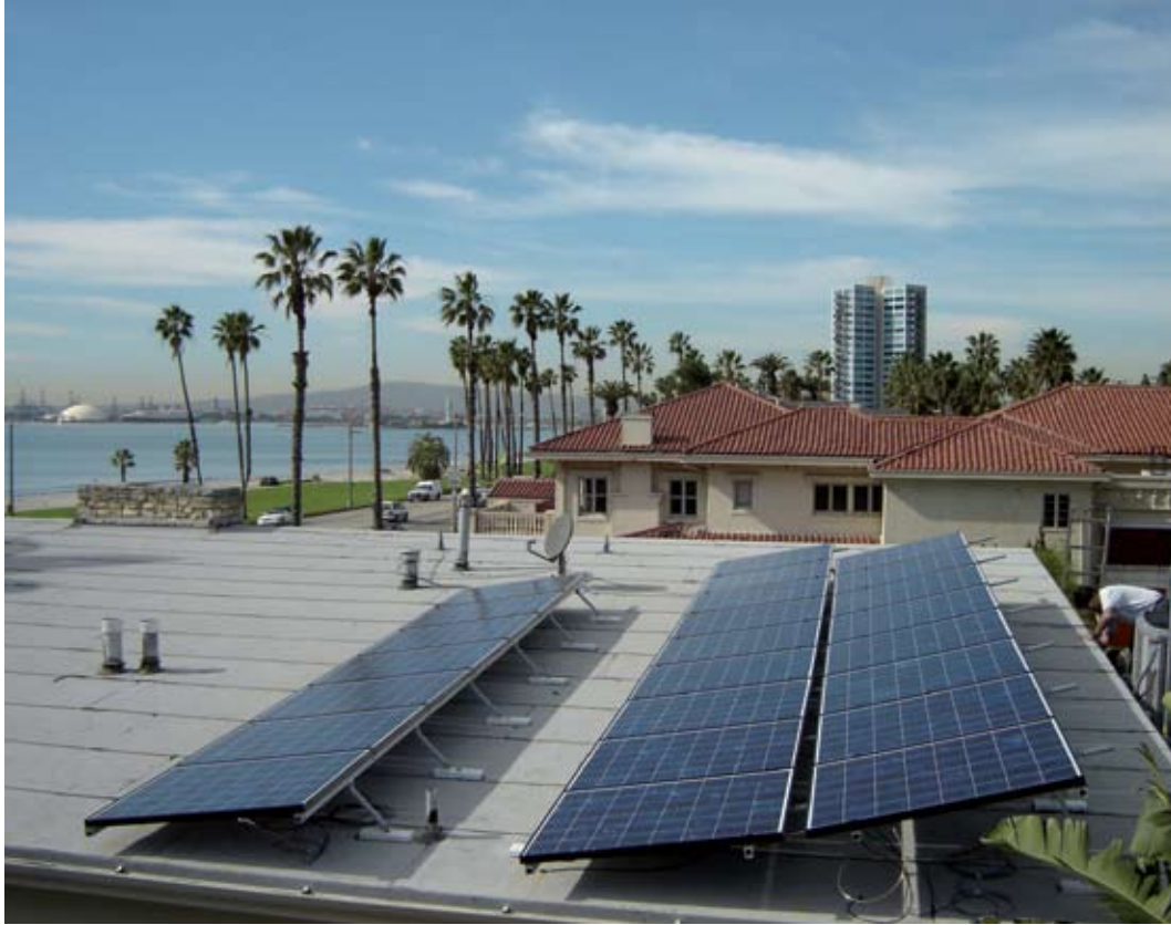
Solar energy systems can benefit all areas of Los Angeles, from the eastside to the west, from the Valley to San Pedro. This solar array creates clean energy against the backdrop of the twin ports of Long Beach and Los Angeles. Credit: Patrick A. Redgate, Ameco Solar
