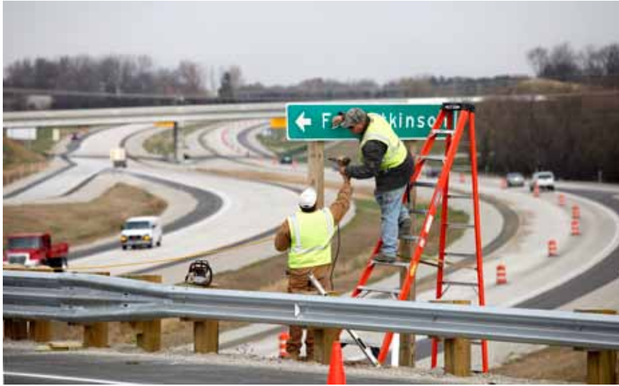
Workers put the finishing touches on the Fort Atkinson bypass, part of the $433 million expansion of State Highway 26.
