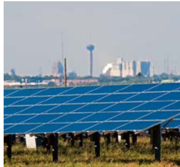
Blue Wing Solar Project in San Antonio, Texas.
