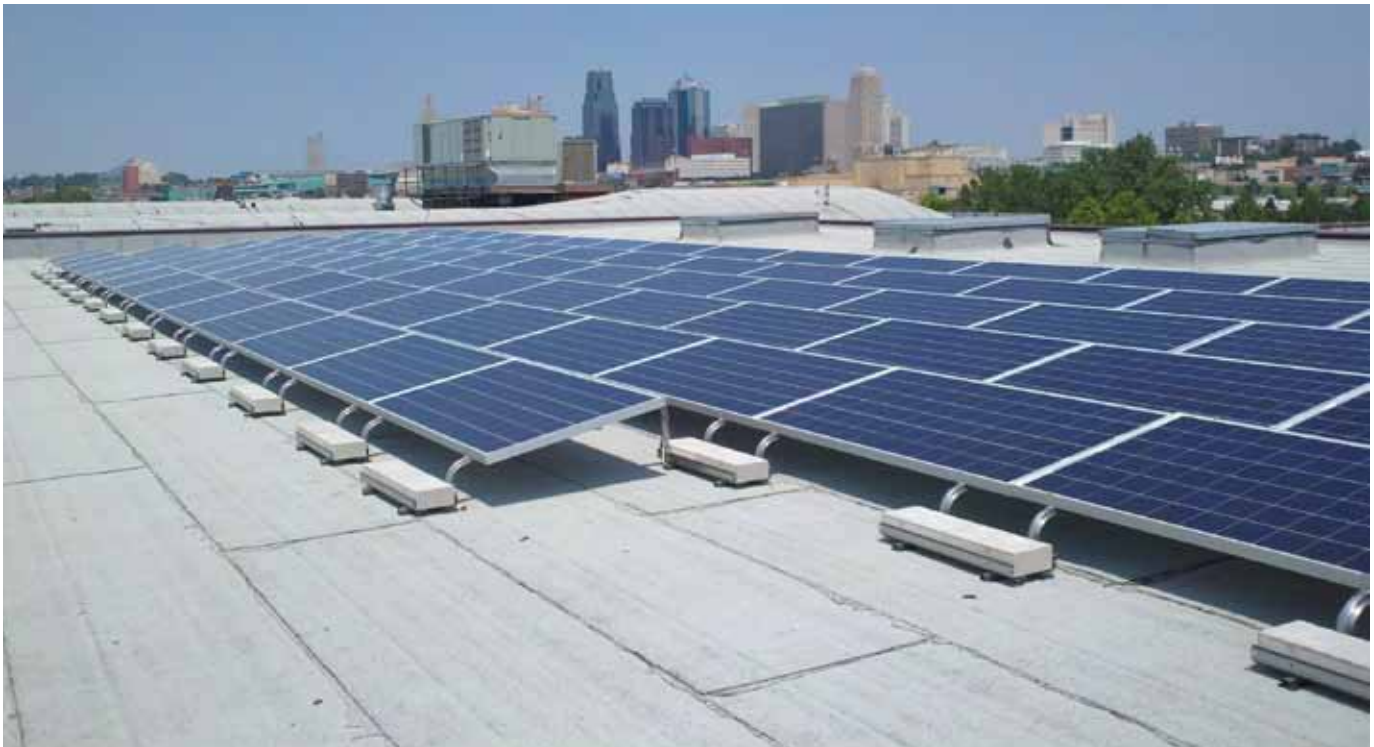
Rooftop solar panels on top of the historic Gem Theater in Kansas City, Missouri.
