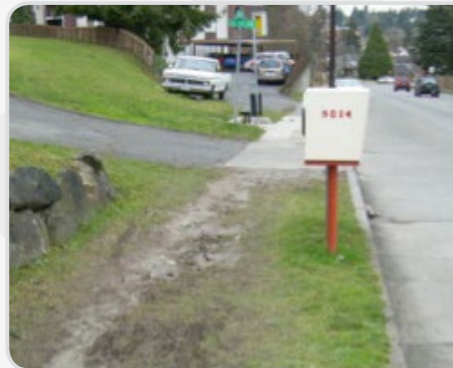
WHERE THE SIDEWALK ENDS: An example of a fractured sidewalk system. Photo: City of Seattle.
