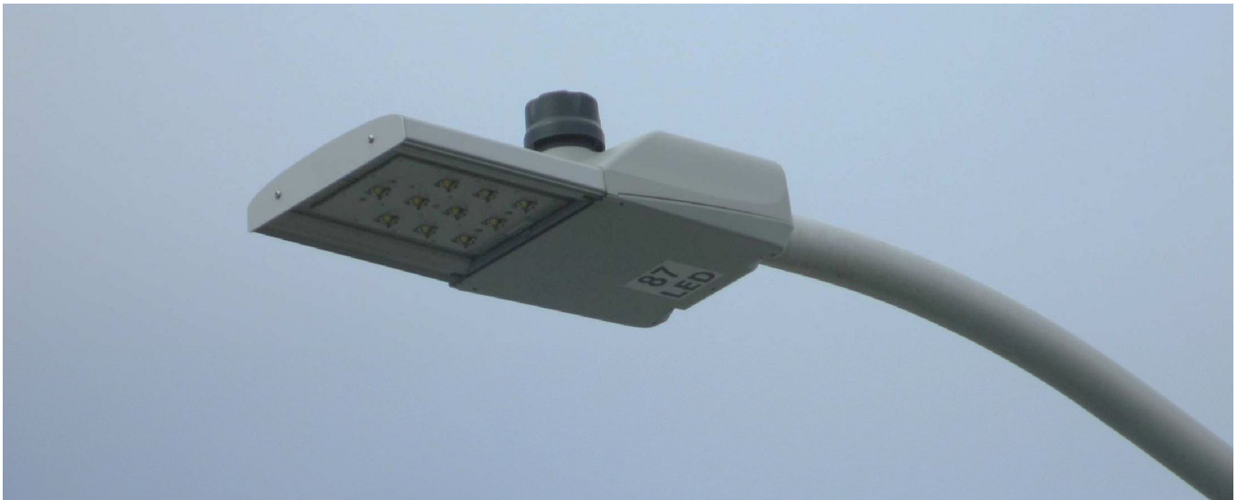
LED streetlights like this one will save the towns of Swampscott and Wenham more than $100,000 in energy costs every year.
