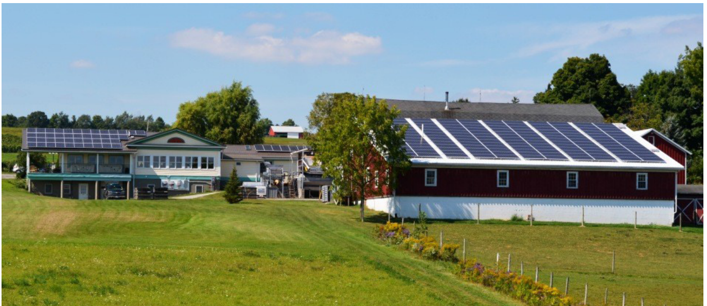
With help from the New York Green Bank, Hunt Country Vineyards installed 348 rooftop solar panels. Credit: Joyce Hunt
