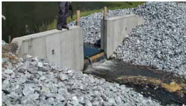
Treated water exiting the Silver Creek acid mine drainage treatment system.
