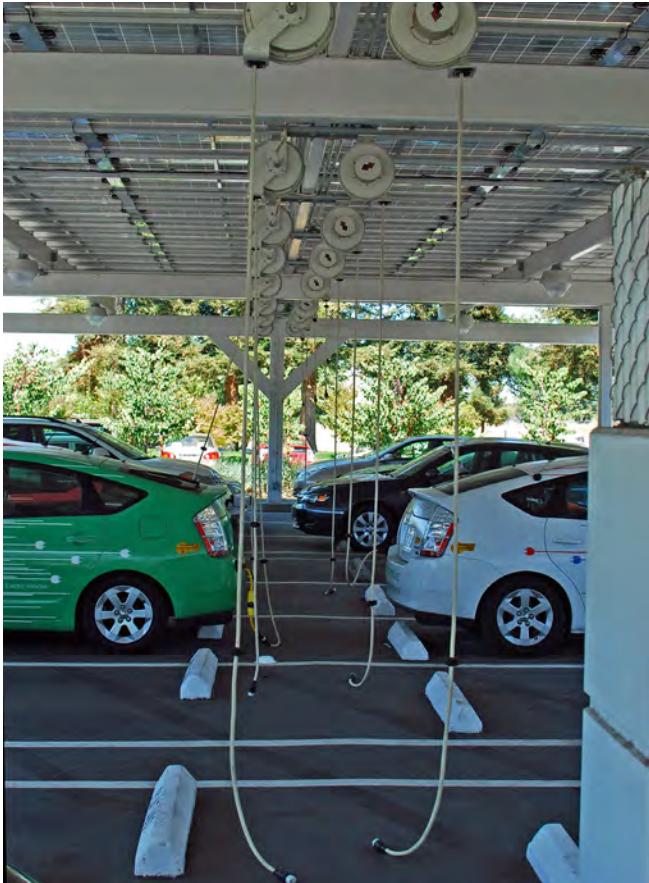
EV charging garage at Google's Mountain View, CA campus. Photo: Nicolas.boullosa, from Flickr, via Wikimedia, CC BY 2.0.
