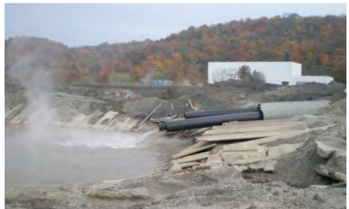
Sluice lines entering “Pond 5” at the J.M. Stuart Station, located in an Ohio River flood zone. Pond 5 was found by an EPA assessment to be in “Poor” condition, and to pose a “Significant” hazard to the surrounding area. Image: EPA
