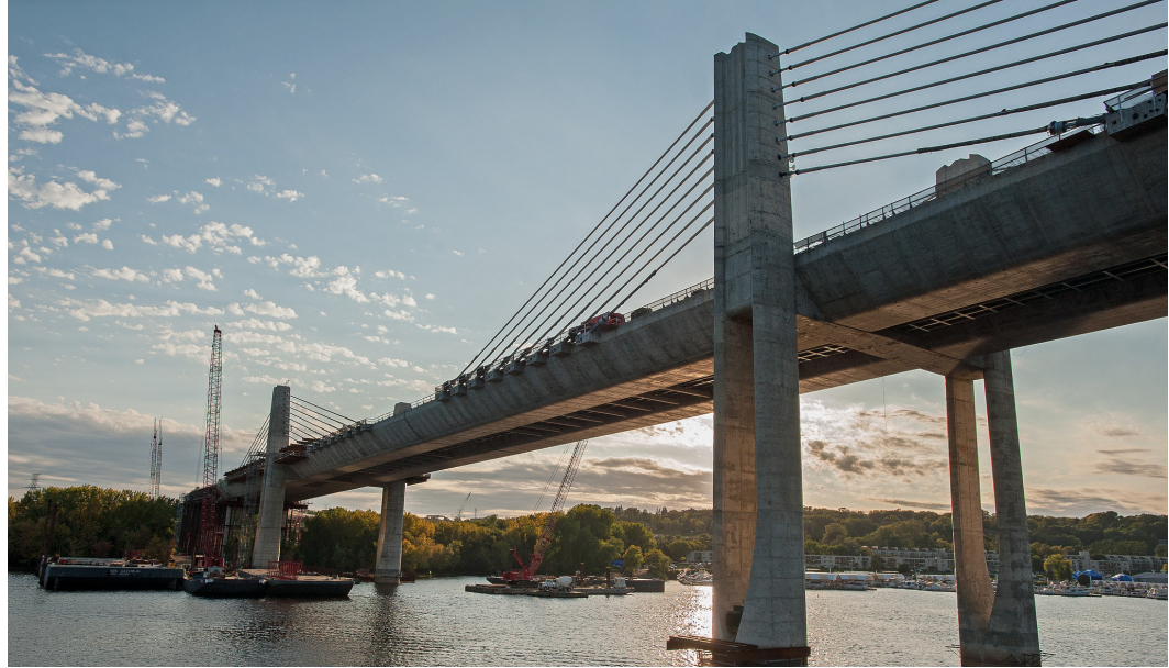
Construction of a new bridge spanning the St. Croix River. Opponents worry it will enable further sprawl. Credit: Minnesota DOT via Flickr, CC BY-NC 2.0.
