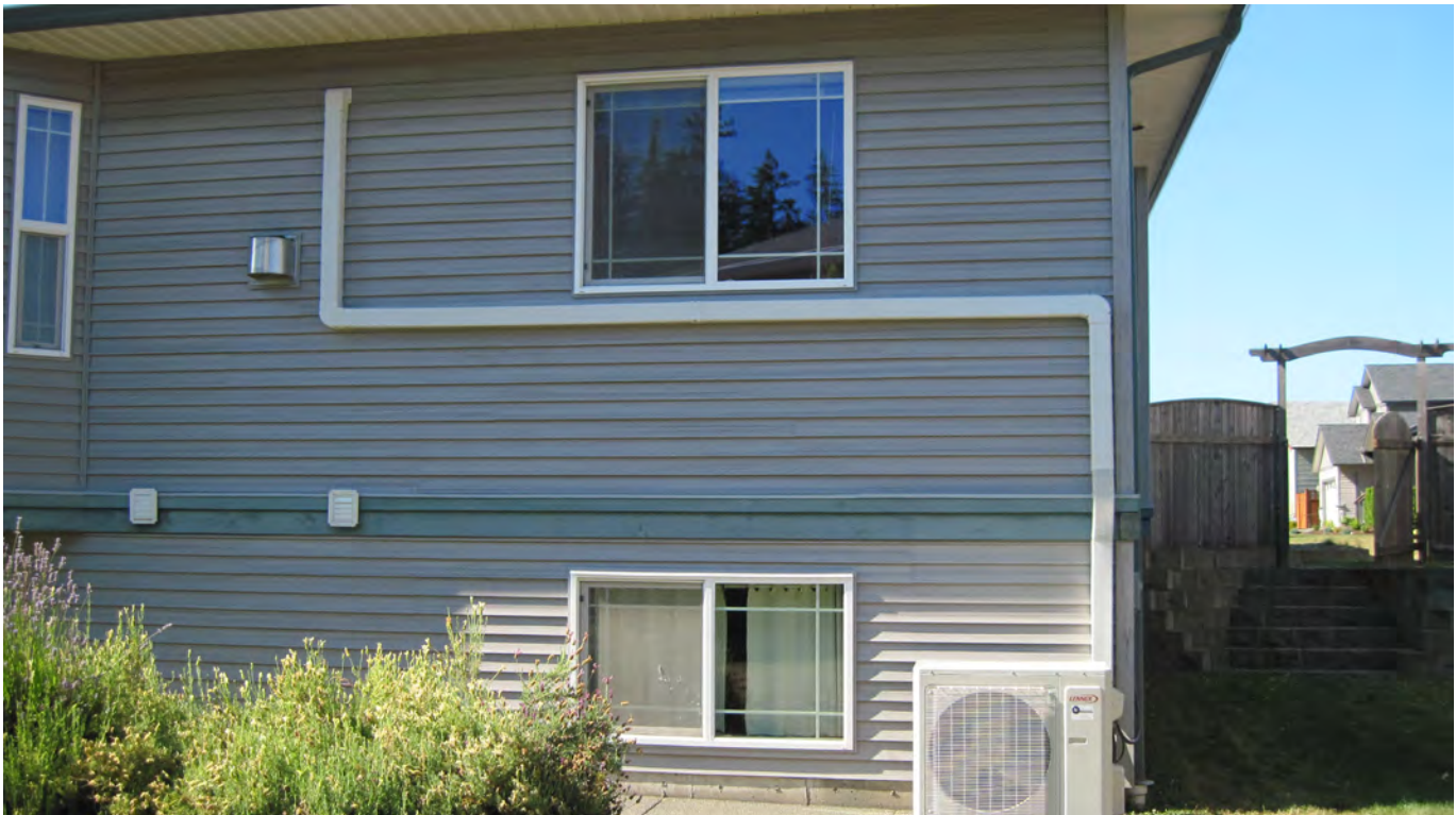
A home with an electric heat pump, which efficiently provides both heating and cooling. Electric appliances such as this, as well as energy efficient design, home batteries and electric vehicles, allow solar panels to meet more of homes' energy needs. Credit: Lani Hudelson via Flickr, CC BY-ND 2.0.
