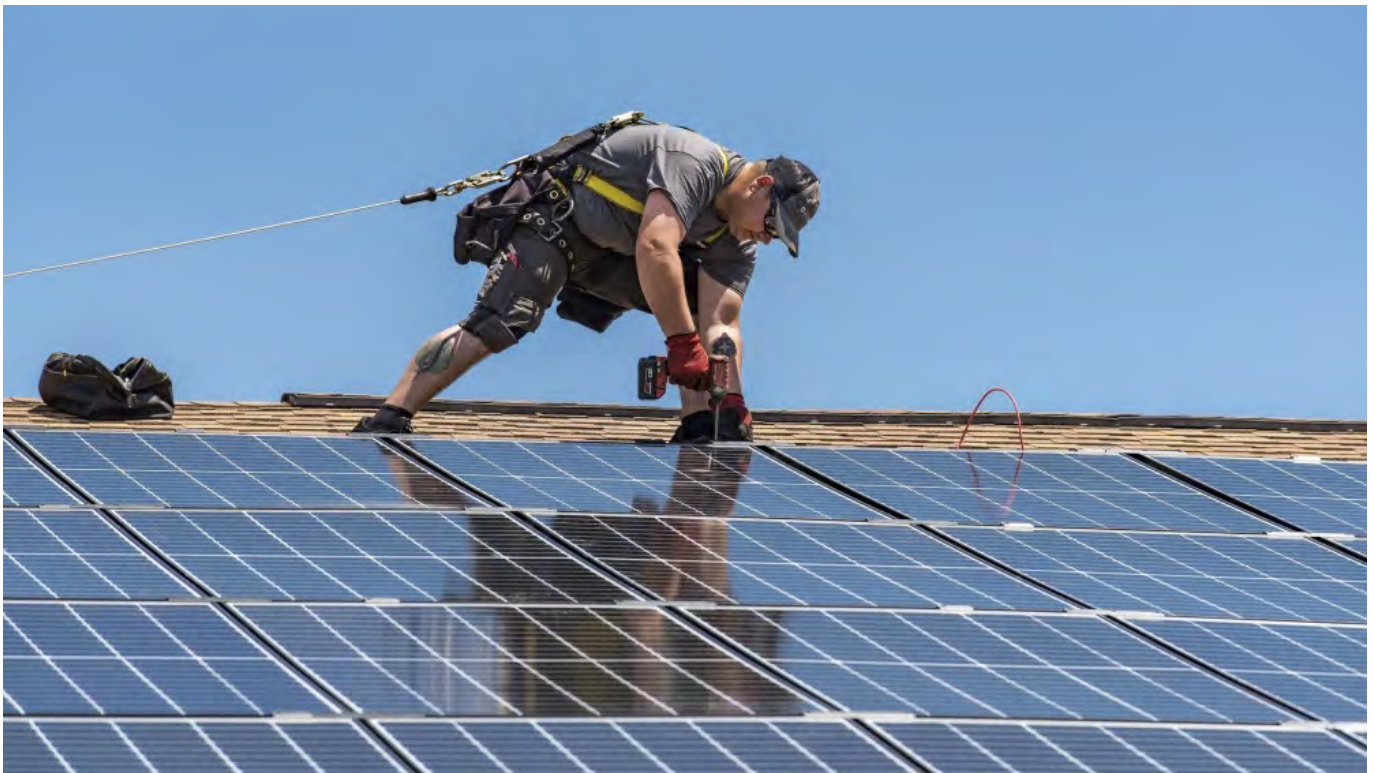
Installing solar PV panels on a home in the Dover Air Force Base in Delaware. Credit: Roland Balik, U.S. Air Force.
