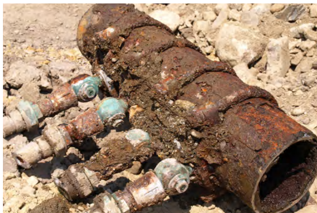
Corroded water main with lead fittings. Photo by Mike Thomas via Flickr, CC BY NC ND 2.0
