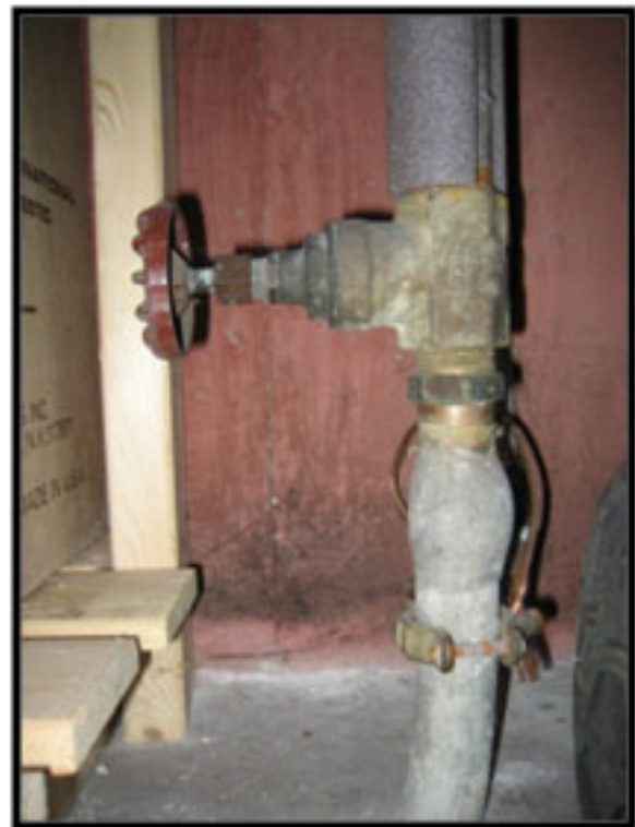
A Lead Service Line 58 Credit: EPA
