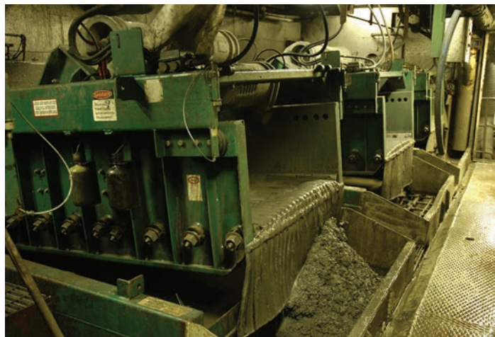
Shale shakers separate drilling mud from drill cuttings, which are one type of waste generated by offshore drilling that may be brought onshore for disposal.
