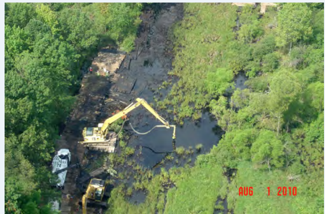
In 2010, a crude oil pipeline spilled 1.2 million gallons of tar sands oil into the Talmadge Creek and Kalamazoo River, requiring a years-long cleanup effort. Image: U.S. Environmental Protection Agency
