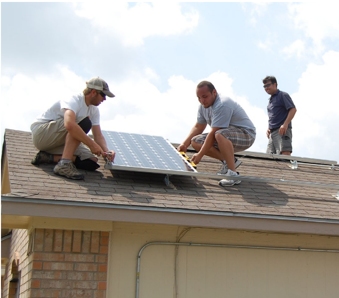
Rooftop solar installation in Del Valle, Texas
