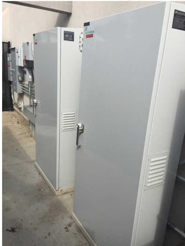
“Behind-the-meter” battery storage at an apartment complex in Los Angeles County, California.
