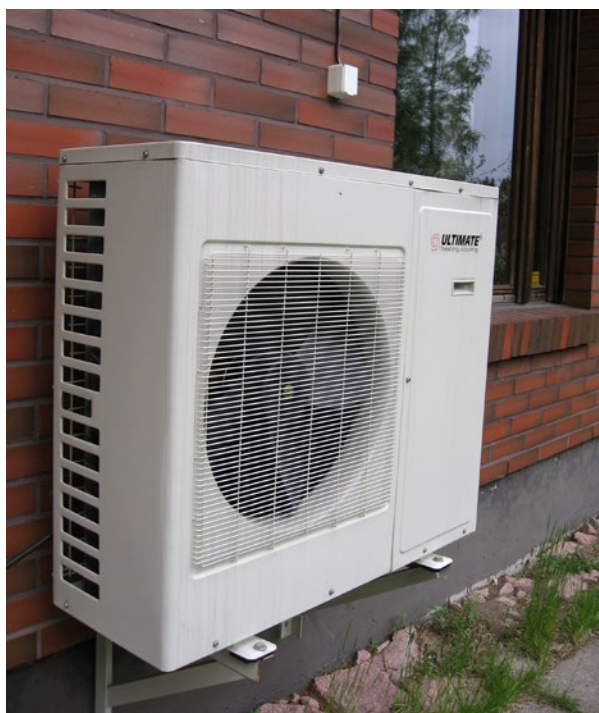
An outside unit of an air-source heat pump.
