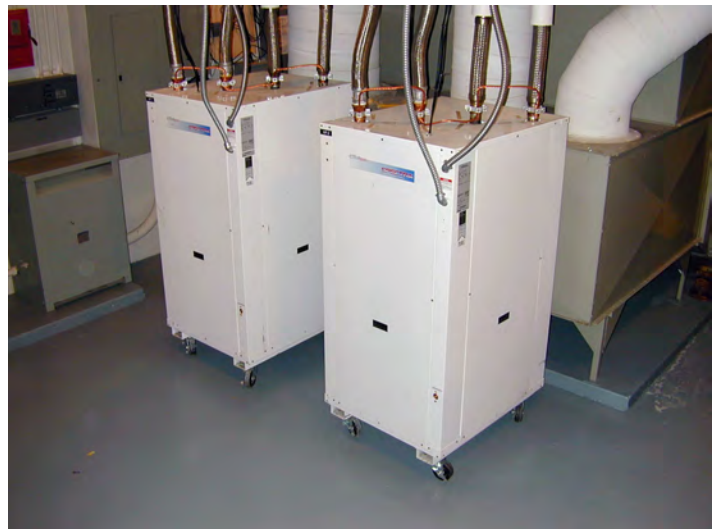
Two 36-ton geothermal heat pumps at the College of Southern Idaho, Twin Falls, Idaho. Photo credit: Bruce Green/NREL
