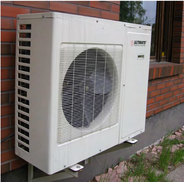
The outside unit of an air-source heat pump. Photo credit: Ppntori via Wikimedia, CC-BY-1.0
