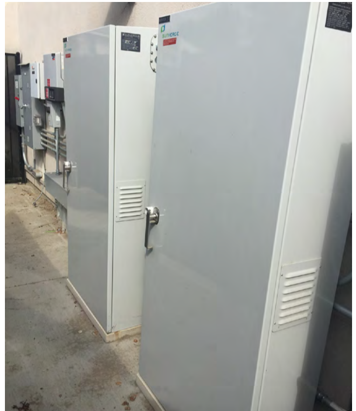
“Behind-the-meter” battery storage at an apartment complex in Los Angeles County, California. Photo credit: Clean Energy Group via Flickr, CC-BY-NC-ND 2.0
