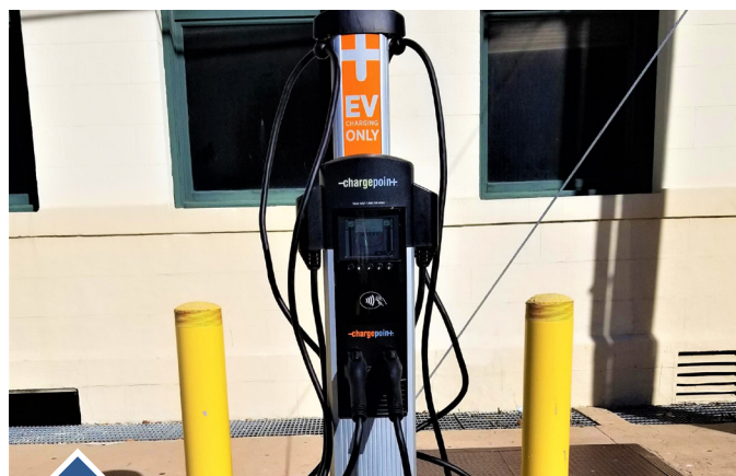
EV charging station in San Marcos.
