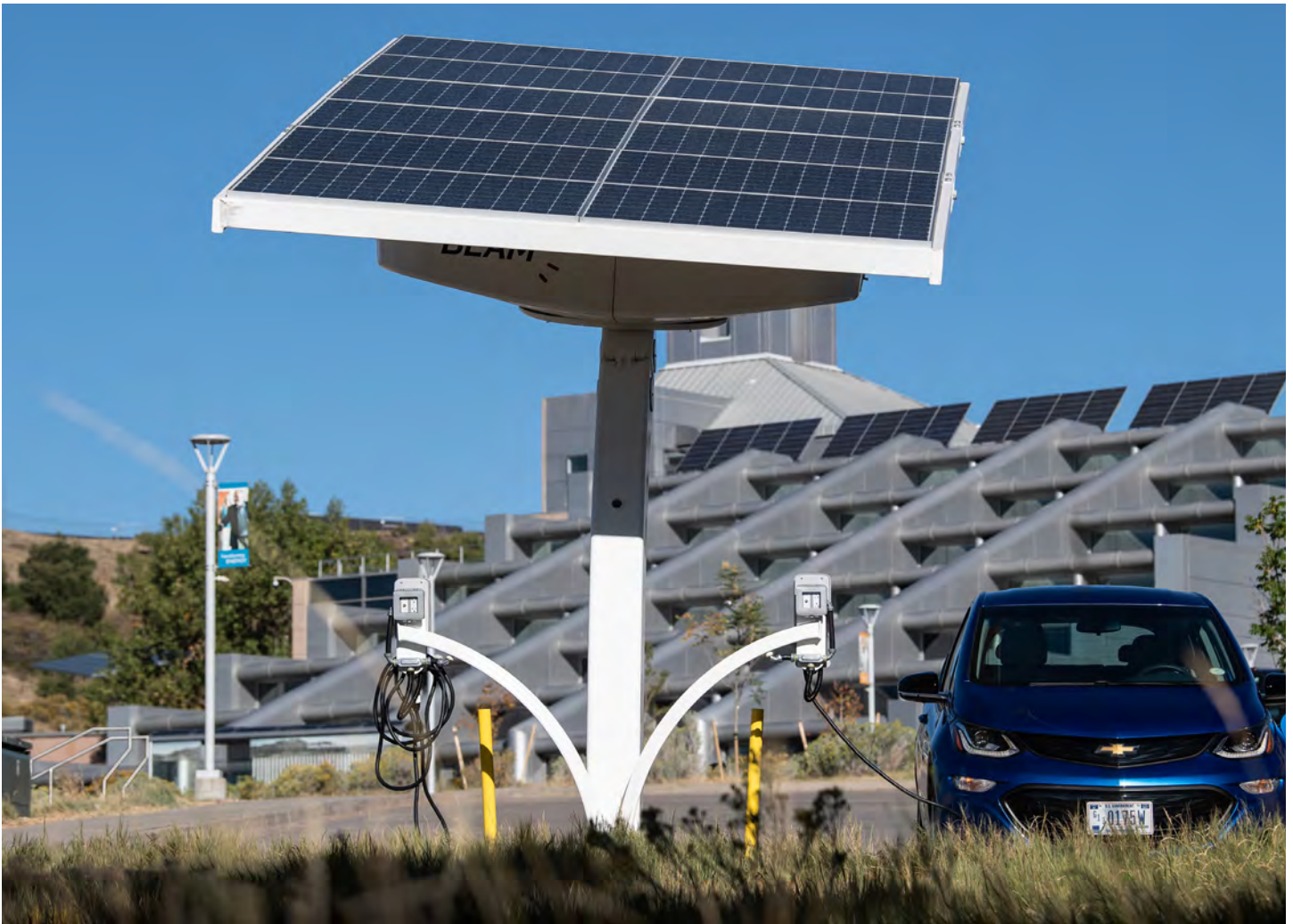
An off-grid, solar powered, solar tracking EV charger in Golden, Colorado. Credit: U.S. Department of Energy via Flickr
