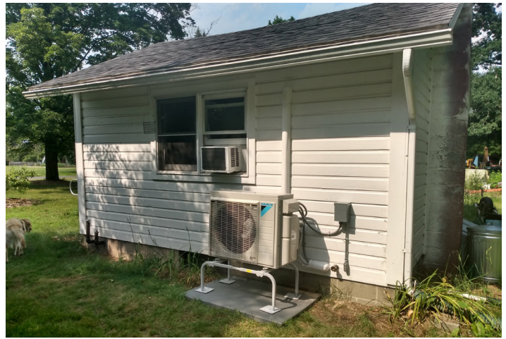
Heat pump outside a home in Amherst, Massachusetts
