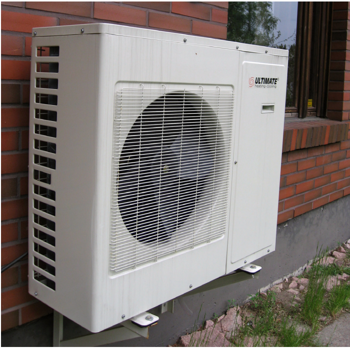
The outside unit of an air-source heat pump. Photo credit: Ppntori via Wikimedia, CC-BY-1.0
