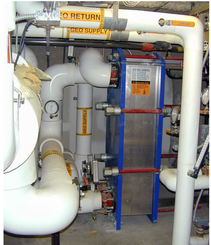
A plate heat exchanger connecting the heating system of the Elks Rehabilitation Hospital in Boise, Idaho to the city's geothermal district heating system. Photo credit: Bruce Green/NREL
