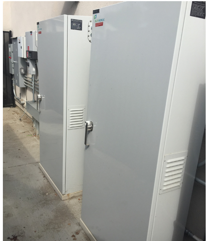
“Behind-the-meter” battery storage at an apartment complex in Los Angeles County, California. Photo credit: Clean Energy Group via Flickr, CC-BY-NC-ND 2.0
