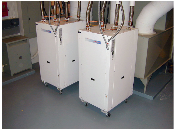
Two 36-ton geothermal heat pumps at the College of Southern Idaho, Twin Falls, Idaho. Photo credit: Bruce Green/NREL
