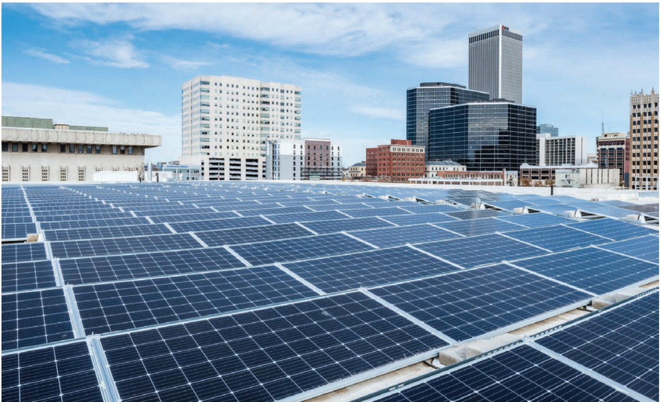
Solar panels overlook the Tulsa skyline from the city's Central Library.
