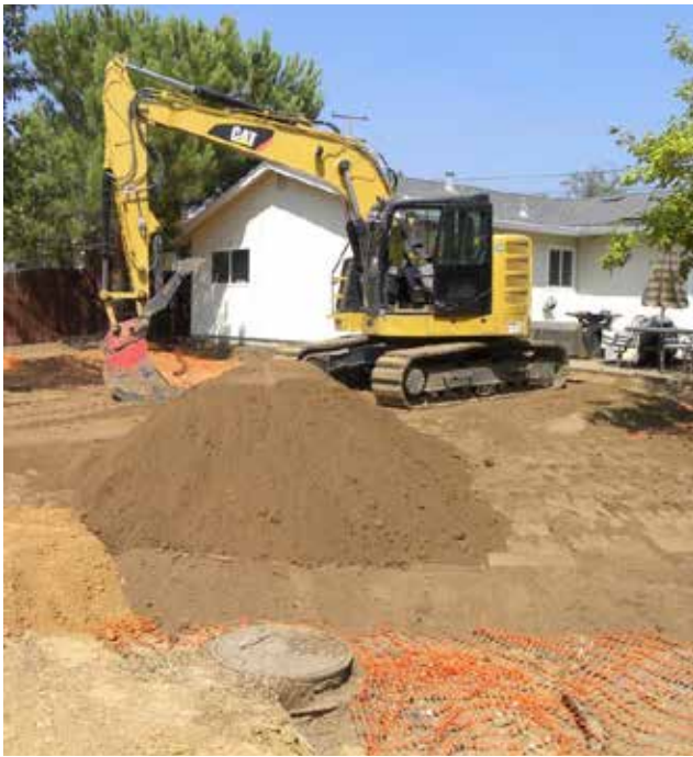
An EPA removal action underway in a residential yard at the Argonaut Mine Superfund Site in Jackson, California. (Source: EPA, On-Scene Coordinator)
