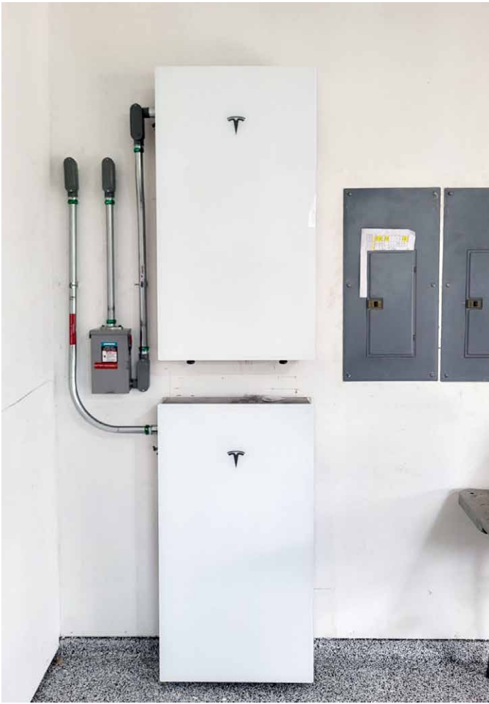
Batteries mounted in a garage can store electricity generated by solar panels on the roof of a home.
