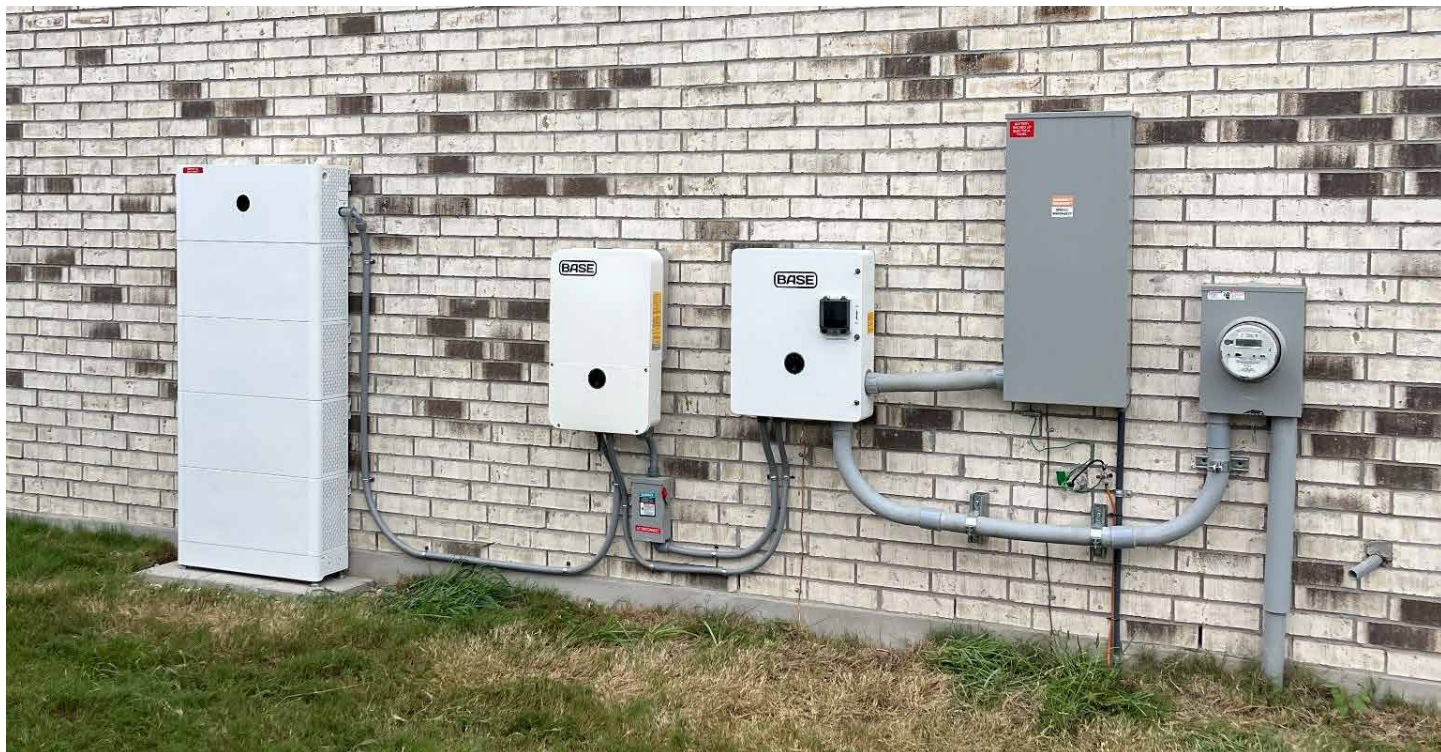
Some components of a solar and storage project. From left to right: a battery, inverter, transfer switch, main electrical panel and electricity meter.
